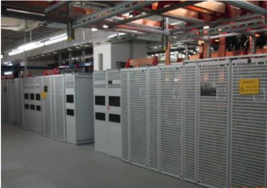
Telekommunikation Flatpack SHE System
